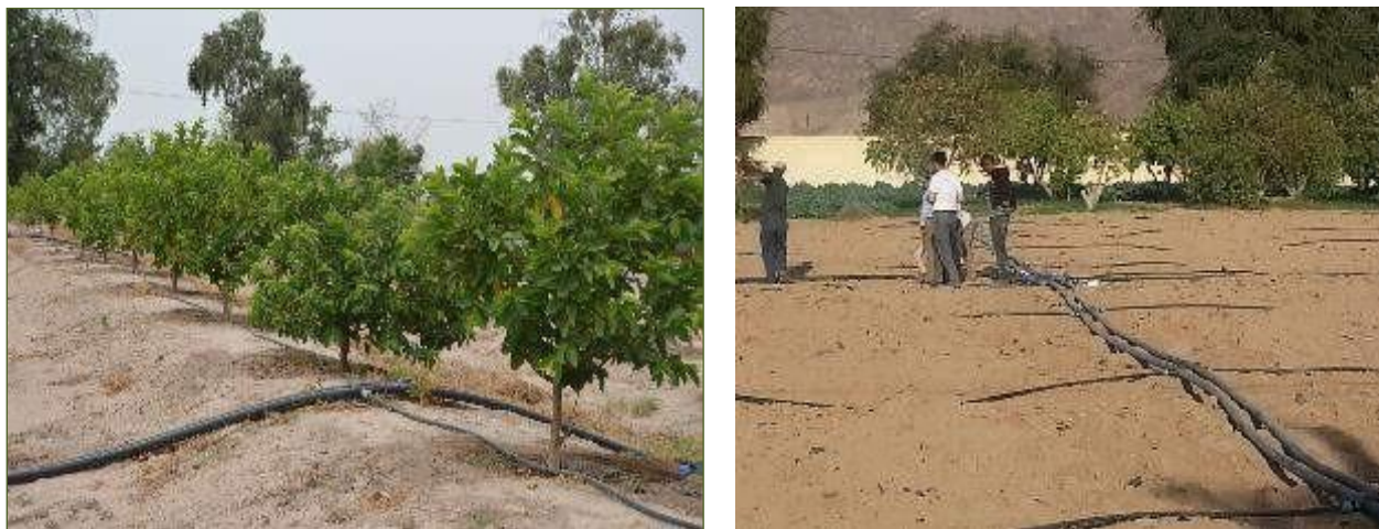
Figure 3: Drip irrigation system used in guava orchards.
